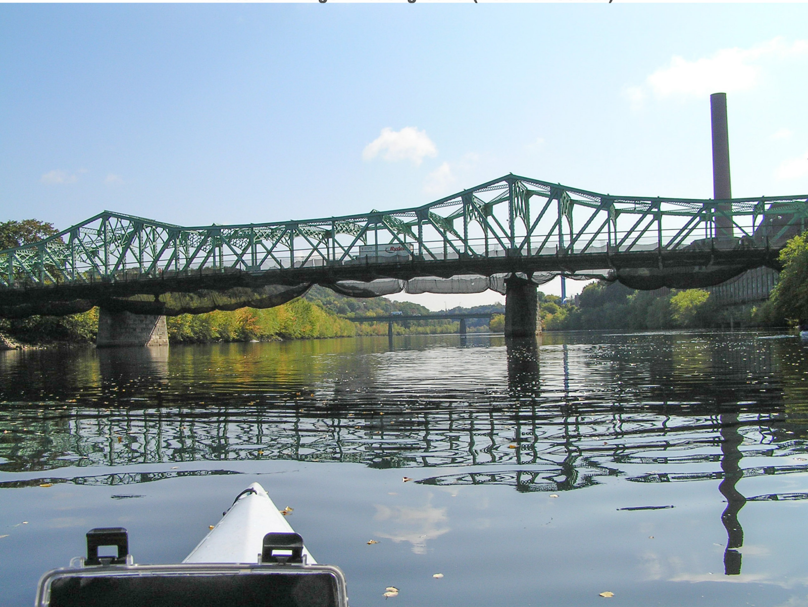
Cox Bridge in foreground (Bridge Street) Year Built - 1937, Structure Length - 144.5 m Route 38 Bridge in background (Nesmith Street)
