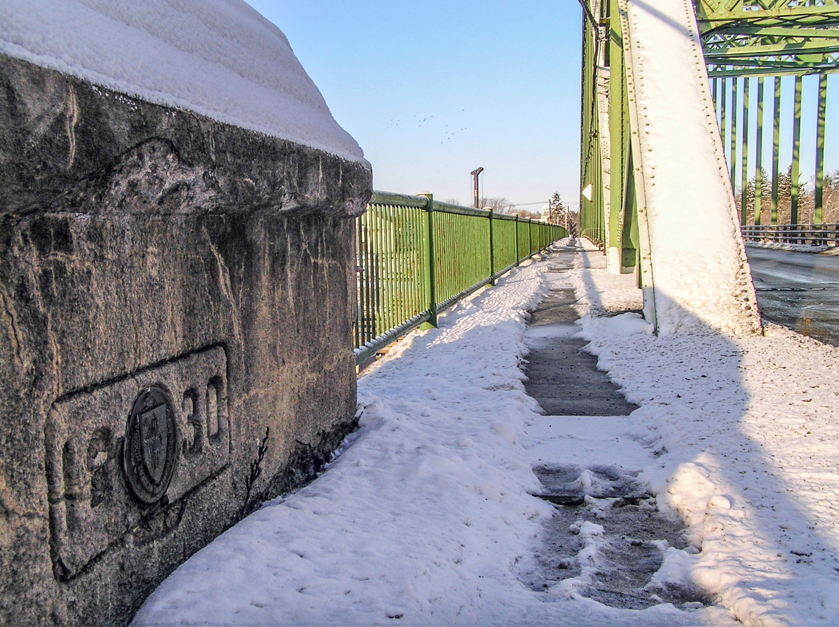
Tyngsboro Bridge showing its age
