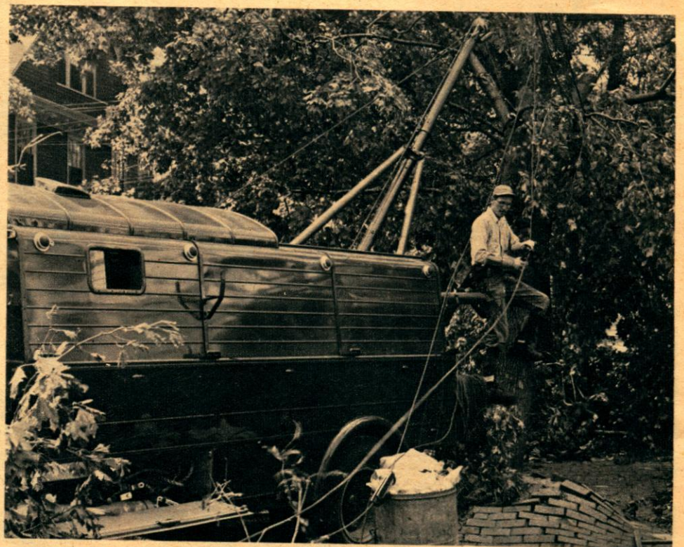
Emergency crews from hundreds of miles away were rushed to the stricken area. Linemen went methodically about the incredible task of unraveling the chaotic snarl of telephone and power lines.
