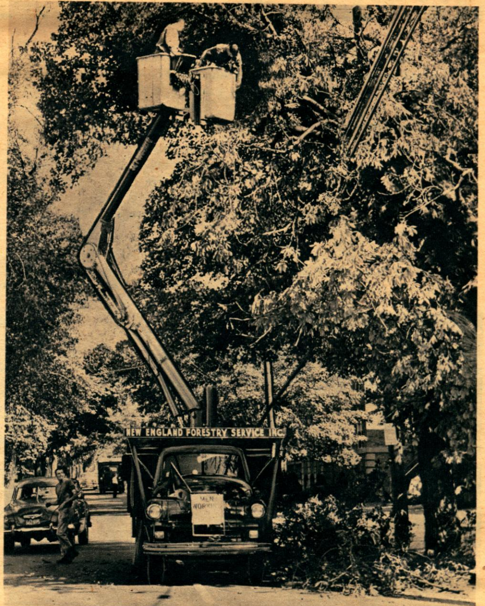
New equipment helped in the heroic battle to restore utilities. This crew of treemen used adjustable "buckets" to untangle the mess in Malden. In this contraption, men could swing themselves right across the street without hindering traffic.
