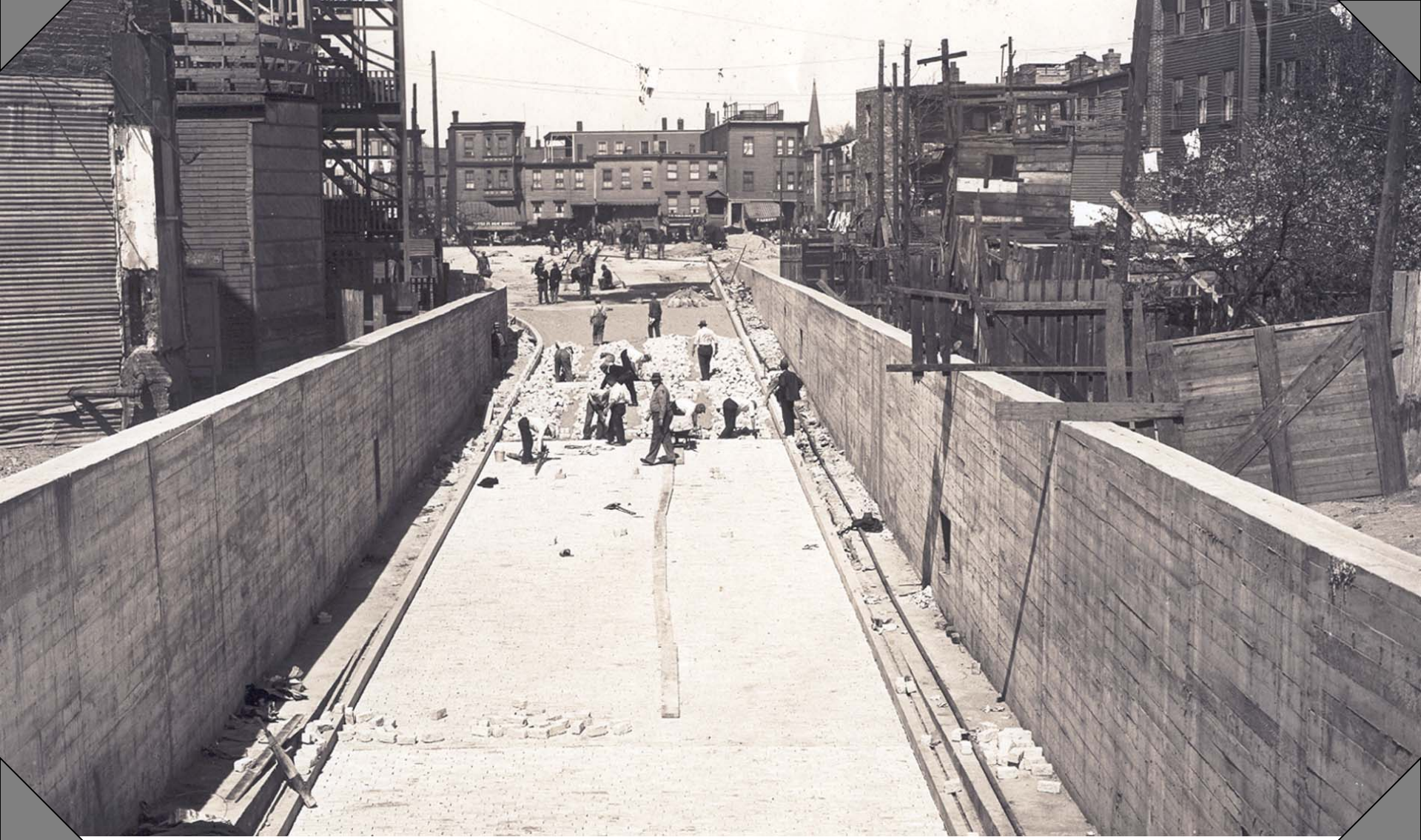
"We furnished the blocks for the Sumner Tunnel. I know we shipped over a million blocks in there." (David Iver Olsson: 1892-1979) Photo says: Paving at the East Boston incline of the Sumner Tunnel, May 4, 1933. Opened in 1934 by the City of Boston, the Sumner Tunnel provided one-lane traffic each way between the North End and East Boston. It wasn't until 1961 that the Callahan Tunnel was opened beside it. The Sumner, owned by the Mass. Turnpike Authority since 1959, exits into the North End and the Callahan exits into East Boston. Fletcher's was on the job here from September 1932 to April 1934. The contract was for $69,500. (A Fletcher Photograph)
